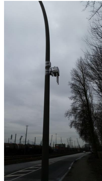
Access Point an Masten
